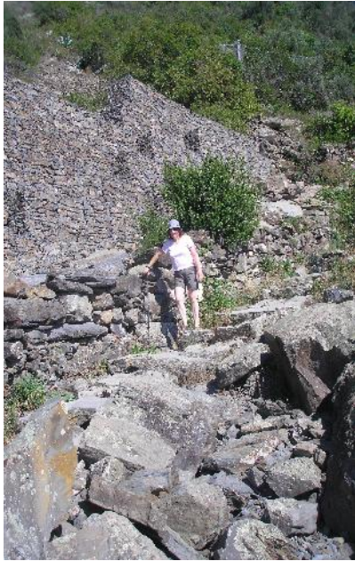
Huge boulders provide evidence of previous heavy rockfalls
